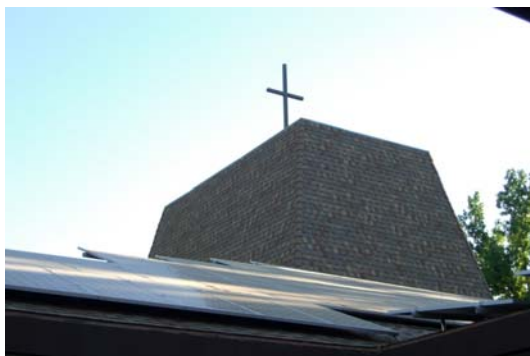
Solar Panels on Church Southern Facing Roof
